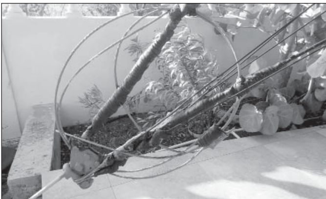
Figure 11 — Fully protected guy wire terminations.
