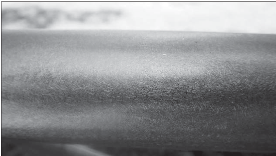
Figure 1 — A close view of a Rohn 55 tower leg after sanding, ready to receive the epoxy primer coat.
