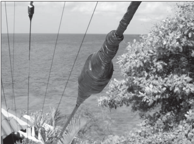
Figure 10 — A Phillystran guy wire, above at the right, connected to a steel EHS cable below, with the insulator and deadends fully potted and protected.
